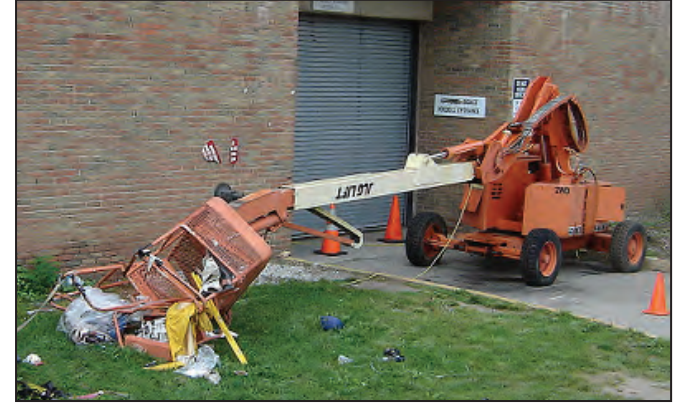
This aerial work platform collapsed during the incident and the lift basket crashed to the ground. (Photo courtesy of OSHA)
