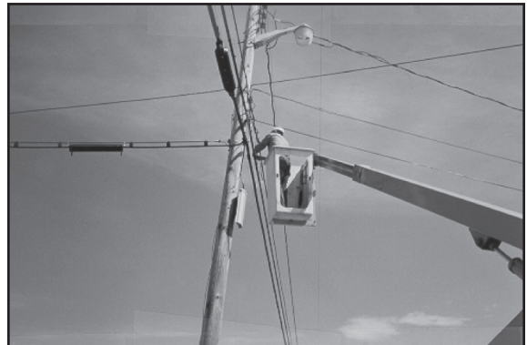
Working without fall protection is dangerous and against OSHA regulations.
