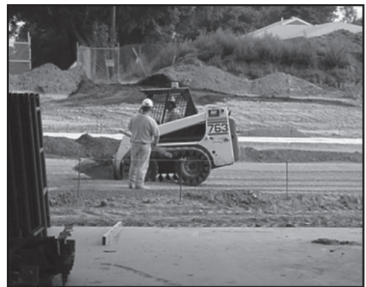
A vest is required for this employee who is in close proximity to the bobcat operator.
