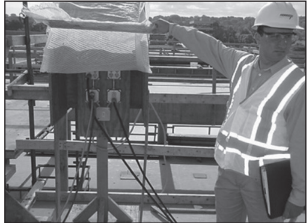
This was a good attempt at providing a weatherproof cover, but wind and rain would likely cause this to fail.
