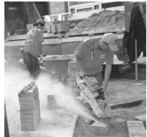
Without dust controls, using a handheld power saw to cut concrete can expose workers to high levels of respirable crystalline silica.
