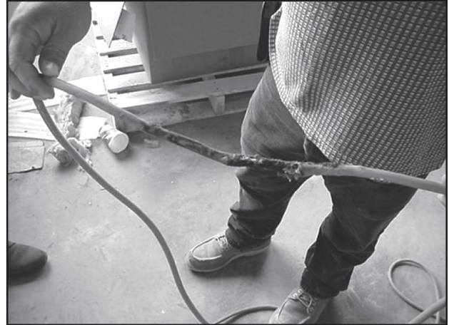
Repair this badly damaged cord with quality dead front plugs or connectors, or replace cord altogether.
