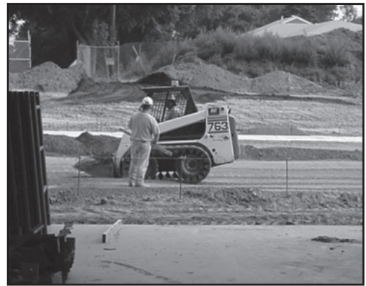
A vest is required for this employee who is in close proximity to the bobcat operator.
