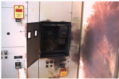
Arc flash in low voltage switchboard cabinet
